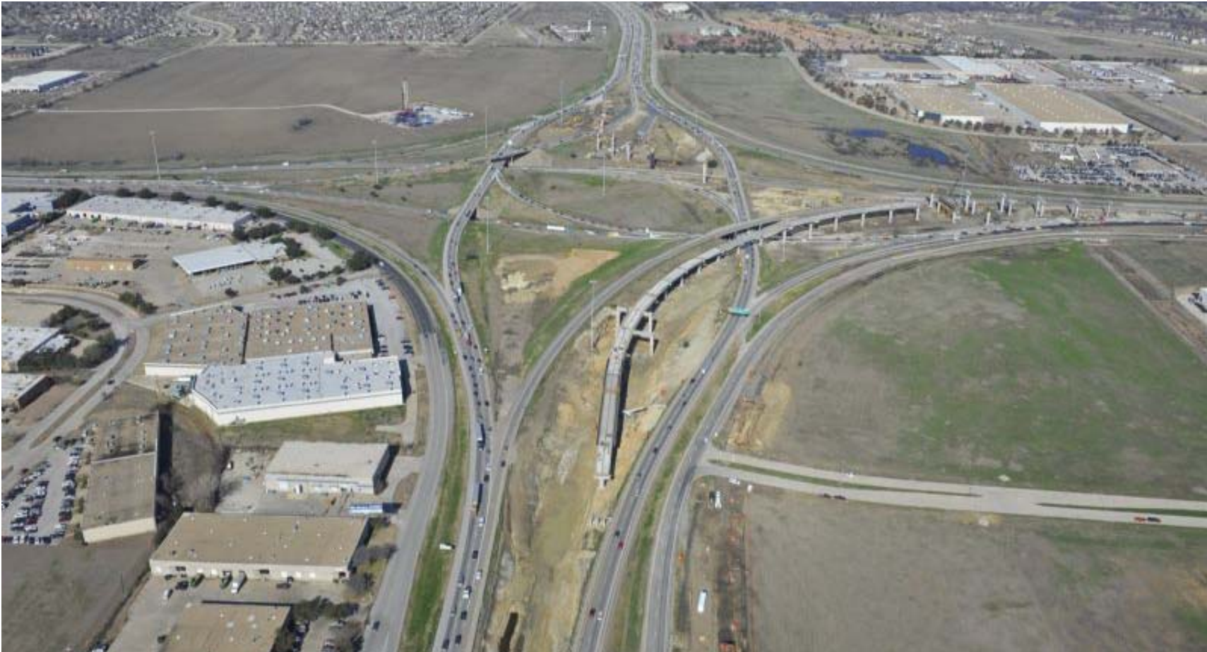
Aerial photograph of the construction progress as of December 2011 on the North Tarrant Expressway near Dallas/Fort Worth, Texas.
